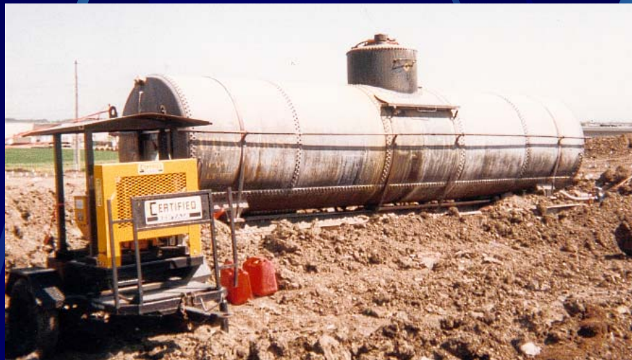
Diesel Generator and Leachate Recovery Tank
